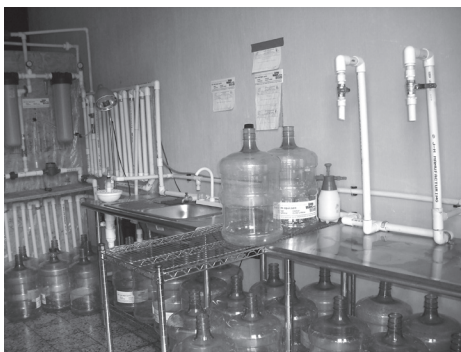
The walk will help add much needed water filtration systems like this one.
